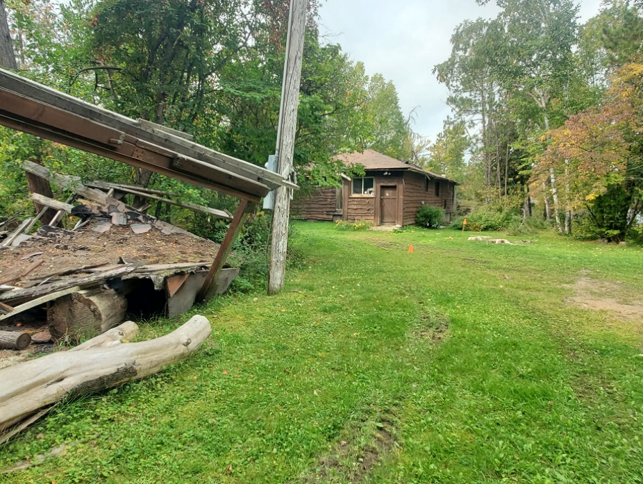
Existing dwelling and collapsed garage
